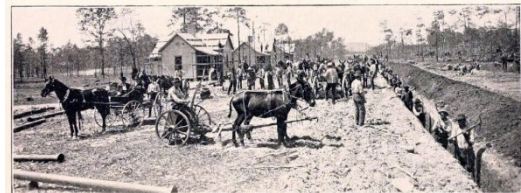
MORELIA AVENUE, OAKWOOD, MAY, 1902. Showing the grading of the street and laying of the eight-inch water main.
